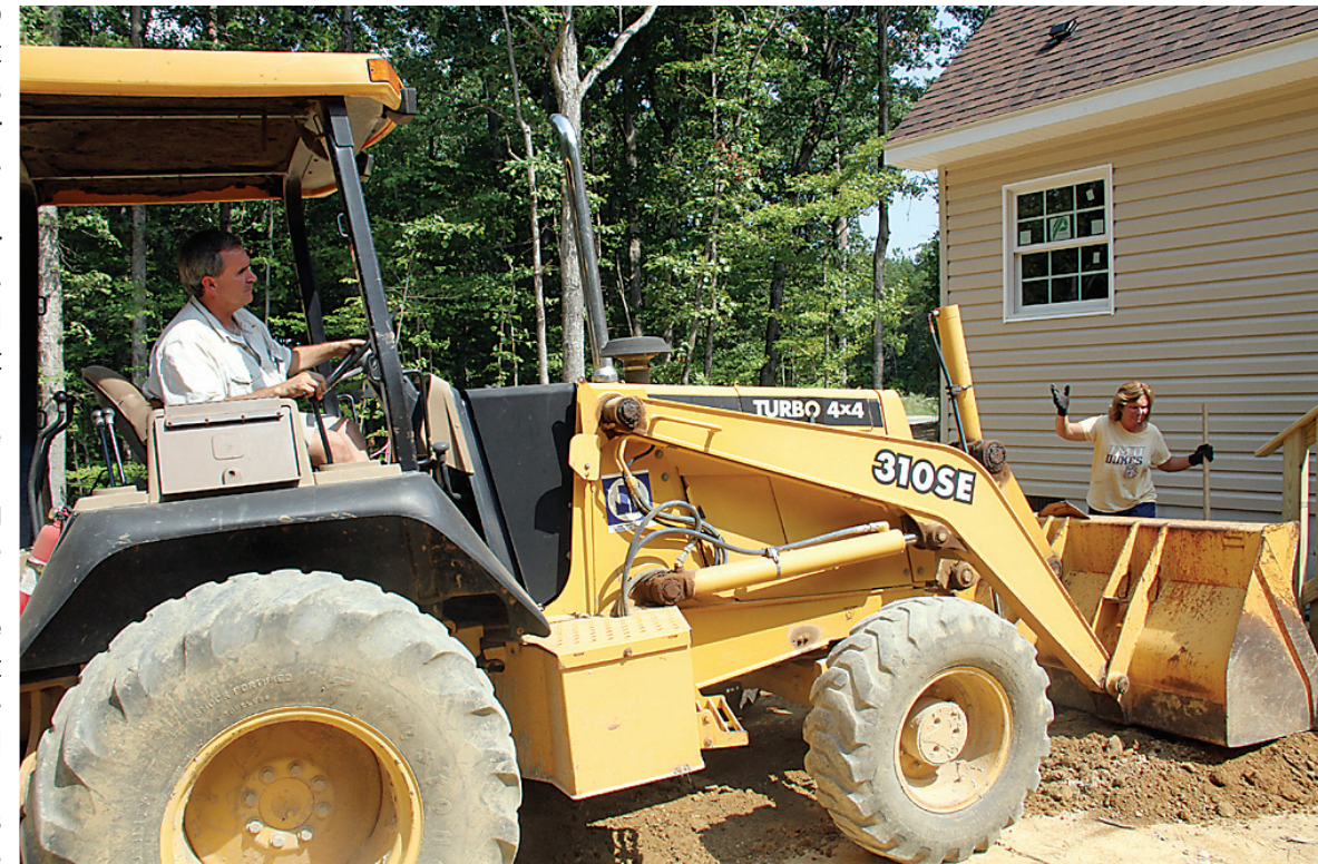
For the past 25 years, Kenny and Lora Dotson have worked side by side, sometimes seven days a week. They are both equally comfortable at the controls of front end loaders, backhoes and bull dozers.
