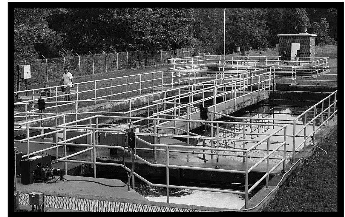
After further purification by trickling filters, effluent meanders through the tanks in the foreground, before being aerated again. In the final tank it is dosed with chlorine and then sulphur dioxide (to remove the chlorine) before heading to the river beyond the small brick building in the background.
