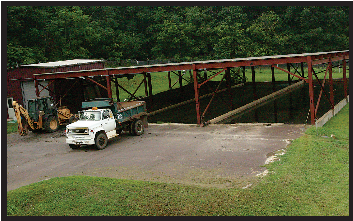
After being treated in the digester for 20 to 30 days, solids are now called sludge and spread out in drying beds under roof before being trucked to the landfill.
