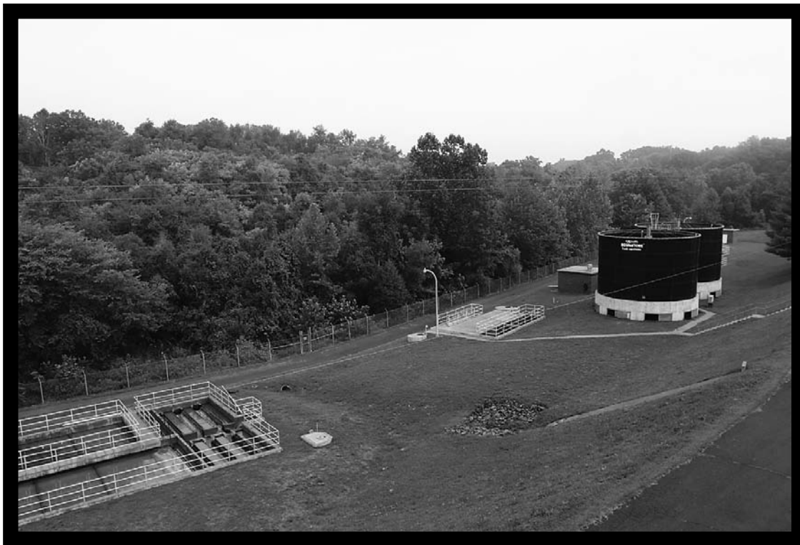
Wastewater flows from the tanks (left) where primary sludge is collected to the trickling filters (right) before eventually being piped to the river.
