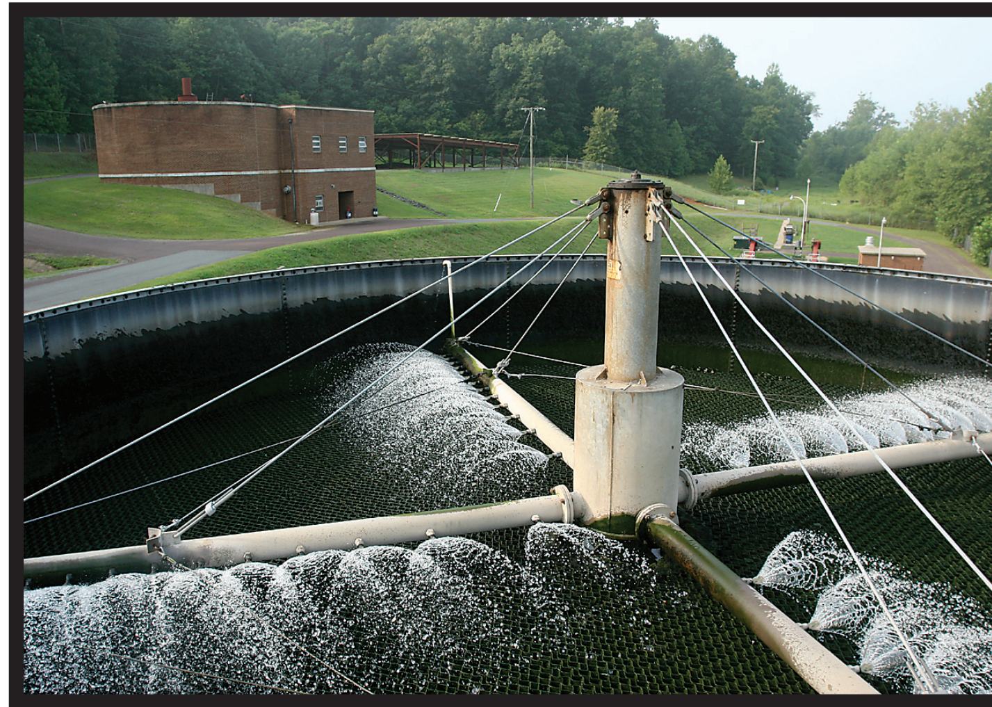
The Orange Wastewater Treatment facility off of Spicer's Mill Road. In the foreground is one of two trickling filters, spraying effluent over a honeycomb populated by aerobic micro-organisms. The brick structure to the rear is the digester.
